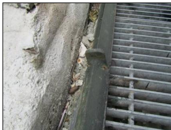
Photos showing the gap between concrete kerb on the track littered with debris and litters
