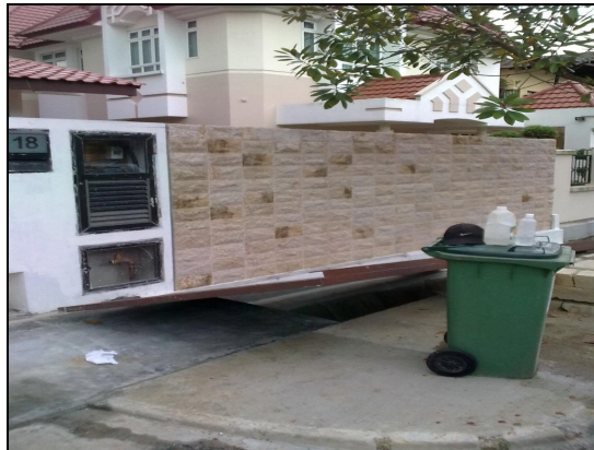
Photo showing the toppled incident gate
