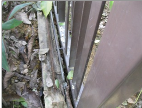
Photo showing the wheels of the incident gate not resting on the track
