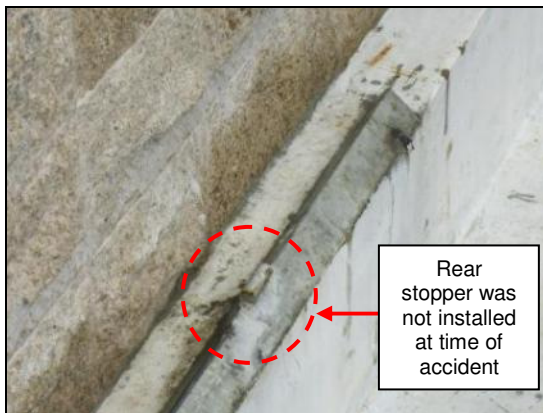
Photo showing the toppled incident gate
